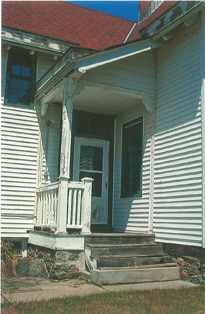
Photo 7. WARWICK NECK KEEPER'S QUARTERS, east entrance, looking west. Existing wood features need to be painted, and stairs repaired.
