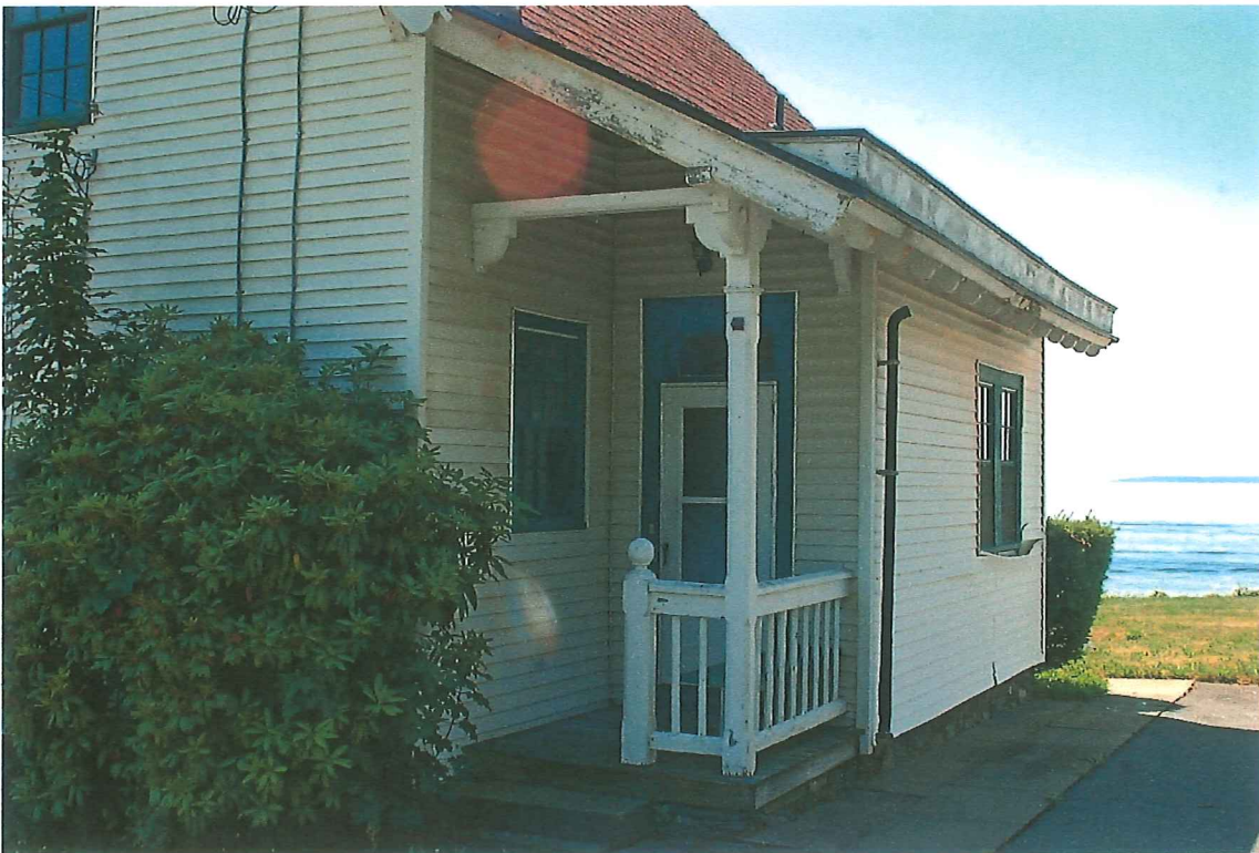
Photo 6. WARWICK NECK KEEPER'S QUARTERS, west entrance, looking southeast. Note, vinyl siding is damaged below windows, downspout is disconnected. These should be addressed as quickly as possible to prevent damage.
