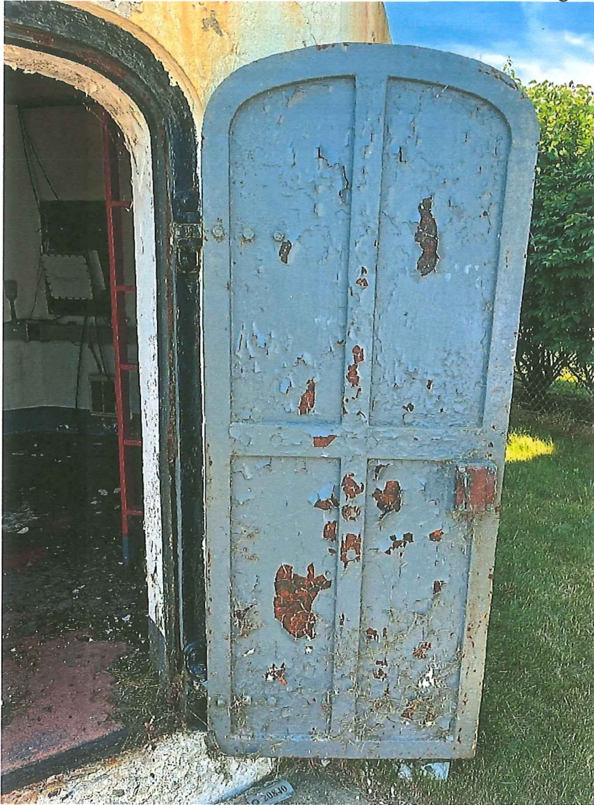
Photo 15. WARWICK NECK LIGHTHOUSE, door detail. Door should be repaired and recoated.
