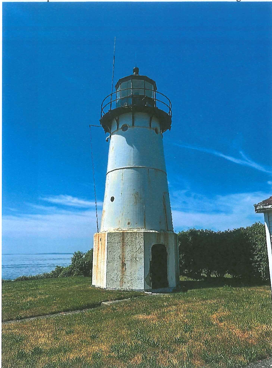
Photo 11. WARWICK NECK LIGHTHOUSE, looking southwest. Lighthouse should be recoated with appropriate paint.
