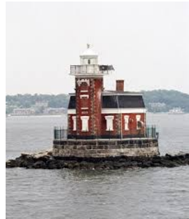
An older photo of Stepping Stones Light, showing the chimney in the rear of the building. This chimney collapsed, leaving a hole in the roof that needed to be repaired. (Photo Credit: USCG)
