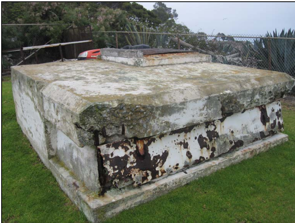
ABANDONED ELECTRICAL TOWER CEMENT
