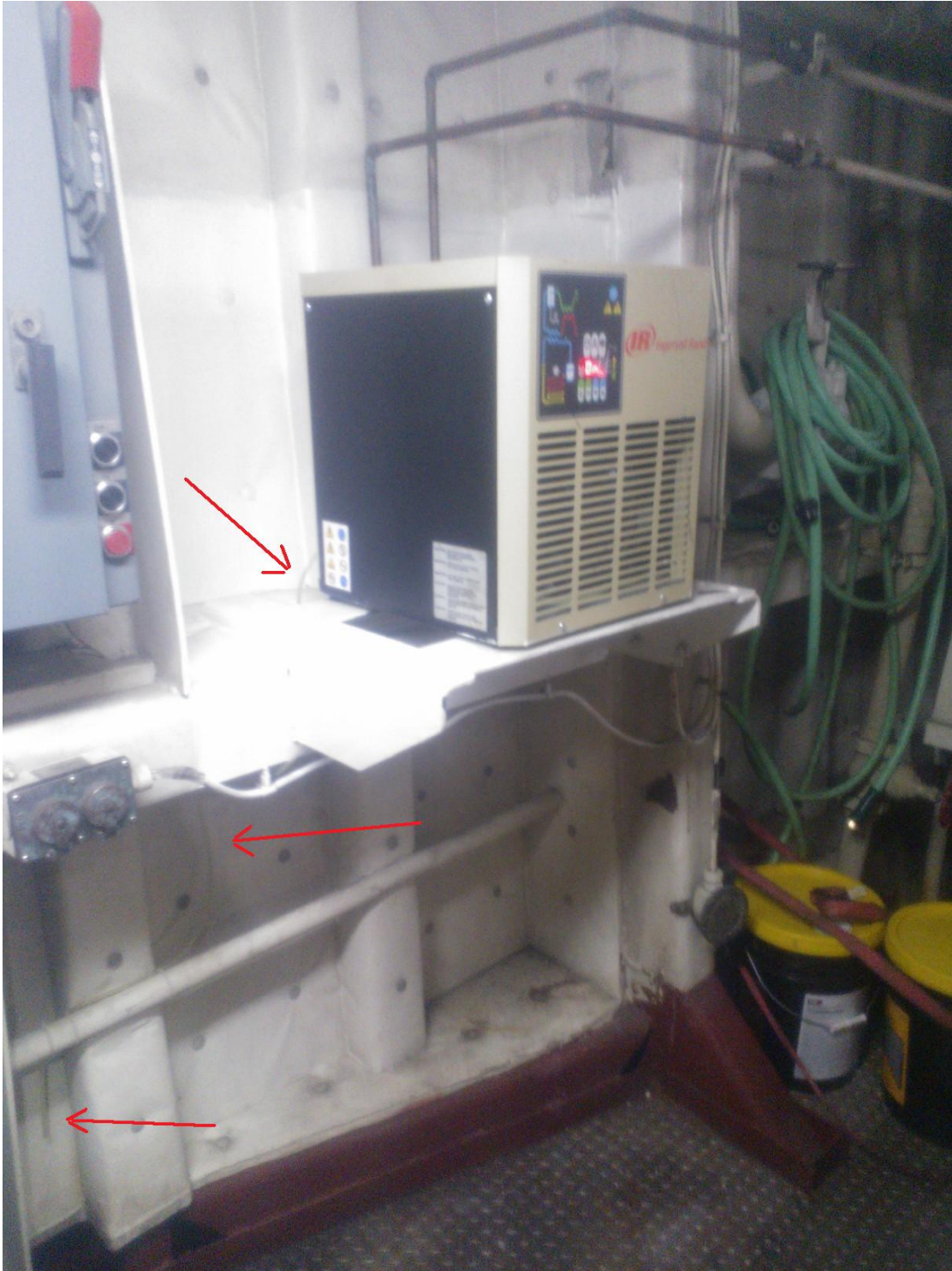
FIGURE 1. NEW AIR DRYER INSTALLED WITH DRAIN LINE IDENTIFIED
