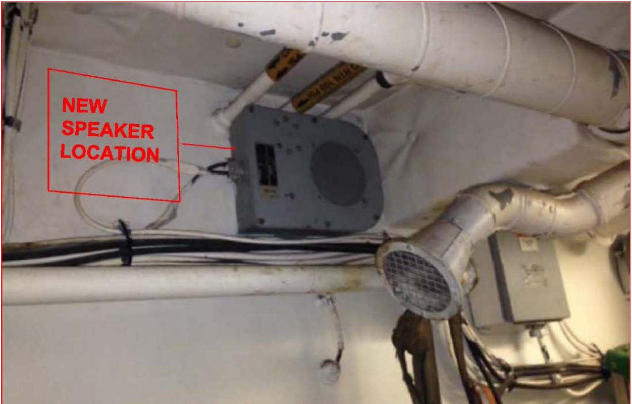
FIGURE 1 – THE 1MC BOX LOCATED RIGHT UNDER AND RUBBED BY HYD. PIPES IN BOASTSWAIN STRM.
